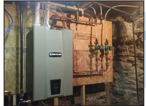
The newly installed WM97+ boiler
