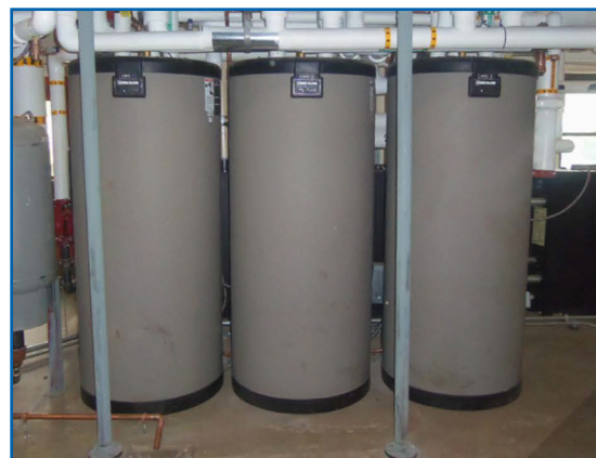
Three new Aqua PLUS indirect fired water heaters installed in the BHA boiler room
