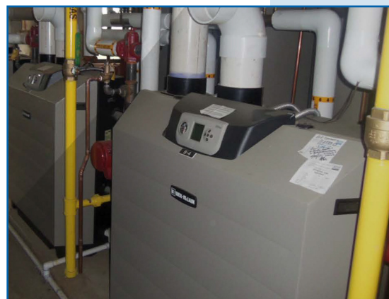
Four new SlimFit 750 boilers installed in the BHA boiler room
